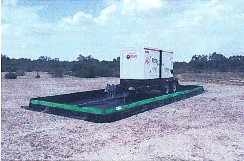
Figure 3: Typical secondary containment barriers for equipment (UltraTech International Inc.)
