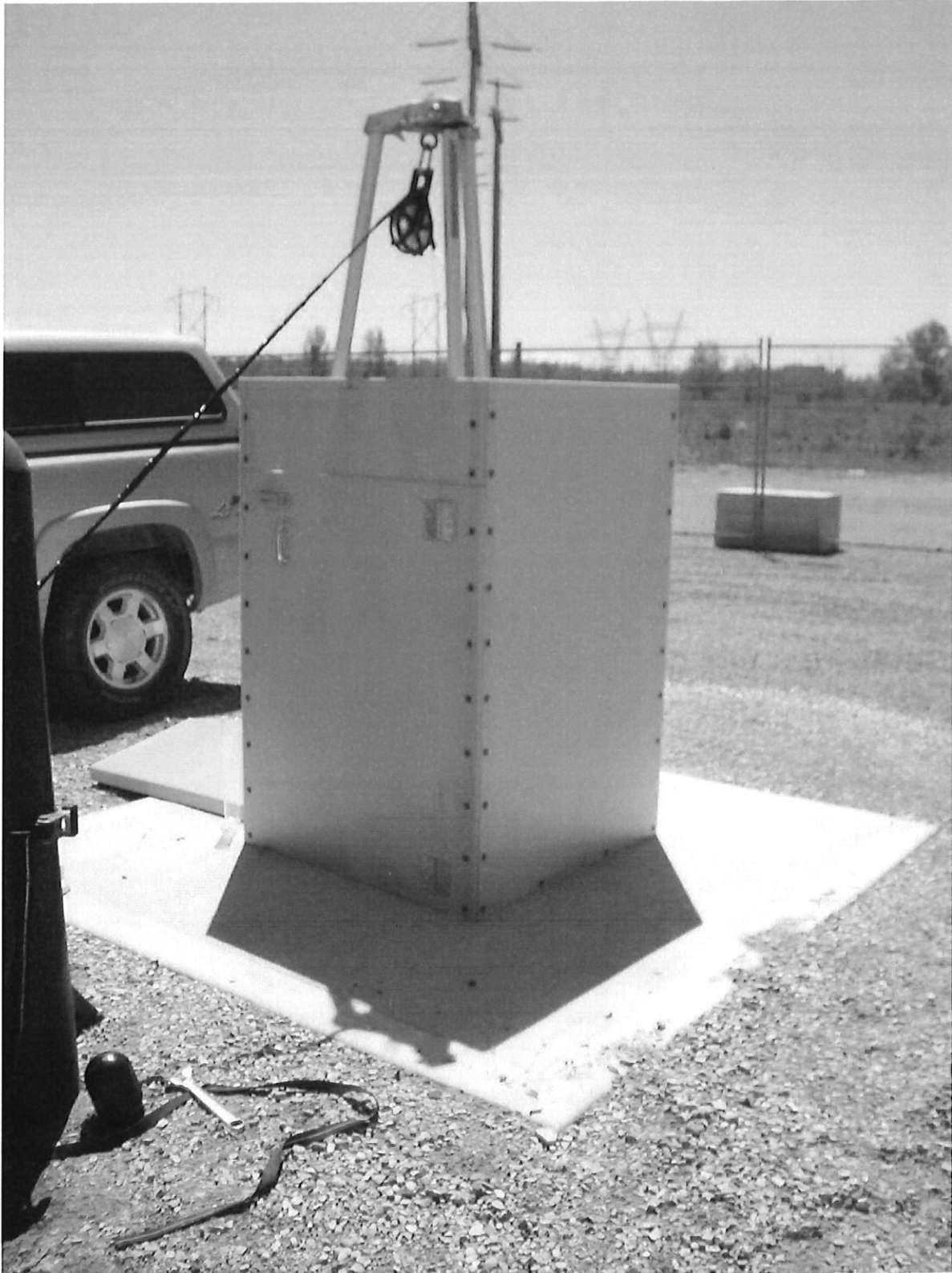
Figure 6: Example of concrete pad with well head enclosure and temporary test equipment.
