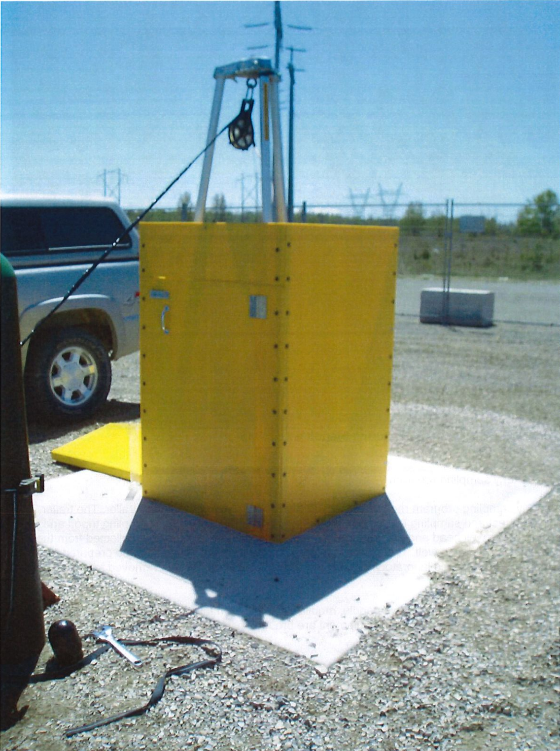
Figure 5: Example of concrete pad with well head enclosure and temporary test equipment.
