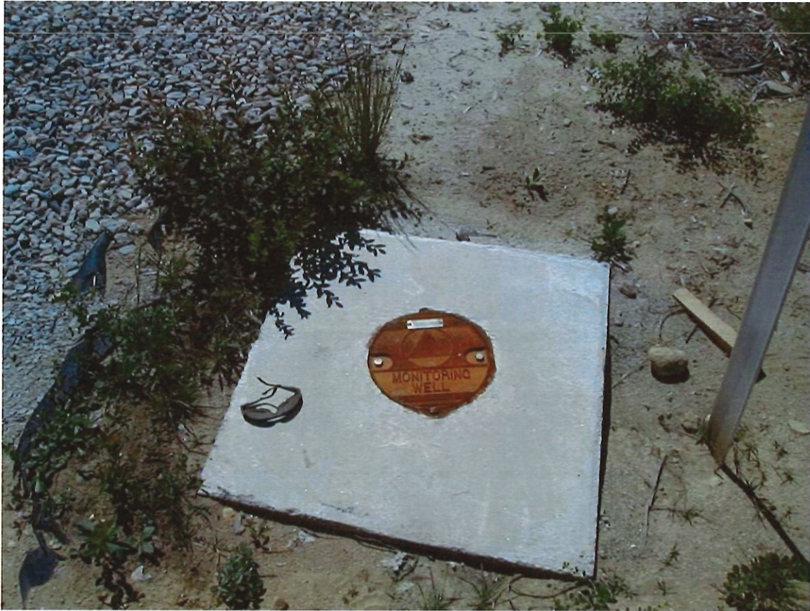
Figure 6: Example of a Monitoring Station with a Cap
