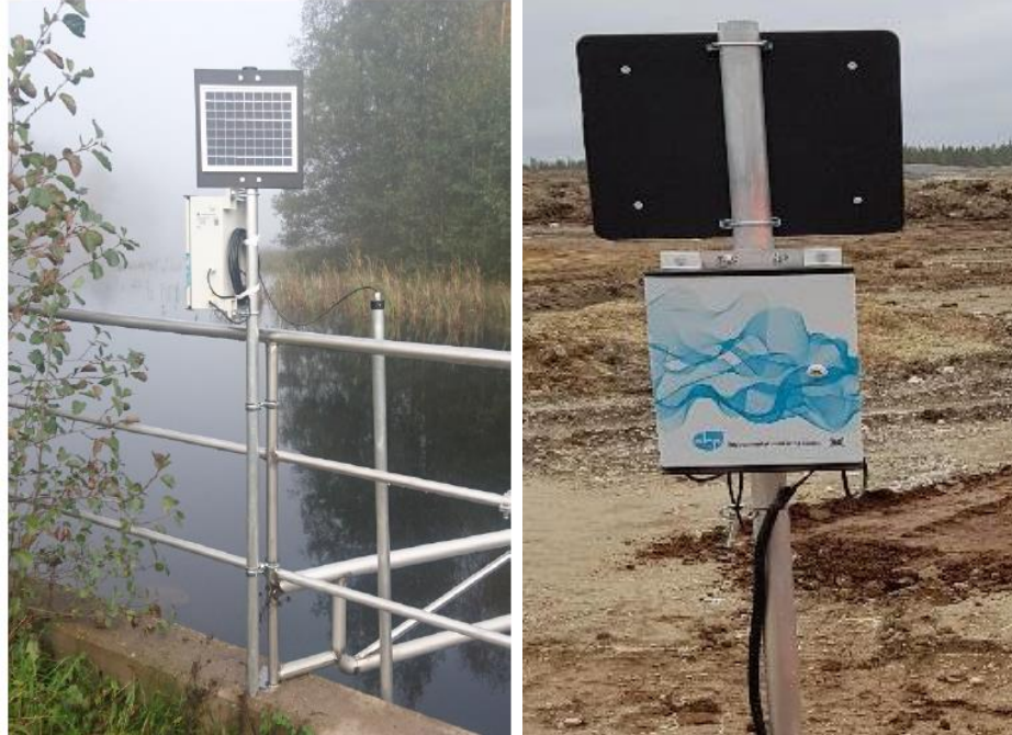
Example pictures of an installation of EHP QMS monitoring station installed to the place of monitoring at industrial site.
