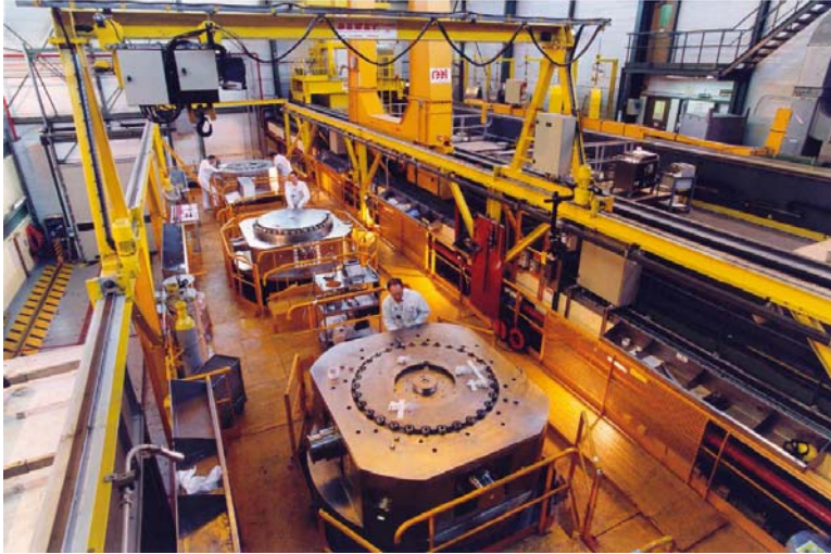
Figure 13. Cask maintenance facility, La Hague, France. (Cogema Logistics Ltd.)
