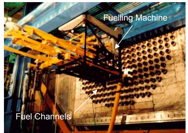
Figure 24. Remote controlled fuelling machine, refuelling a CANDU reactor core.
