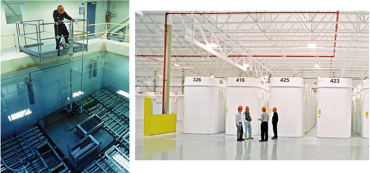
Figure 2.3: Photos of workers in CANDU used fuel bay and in dry storage facility.
